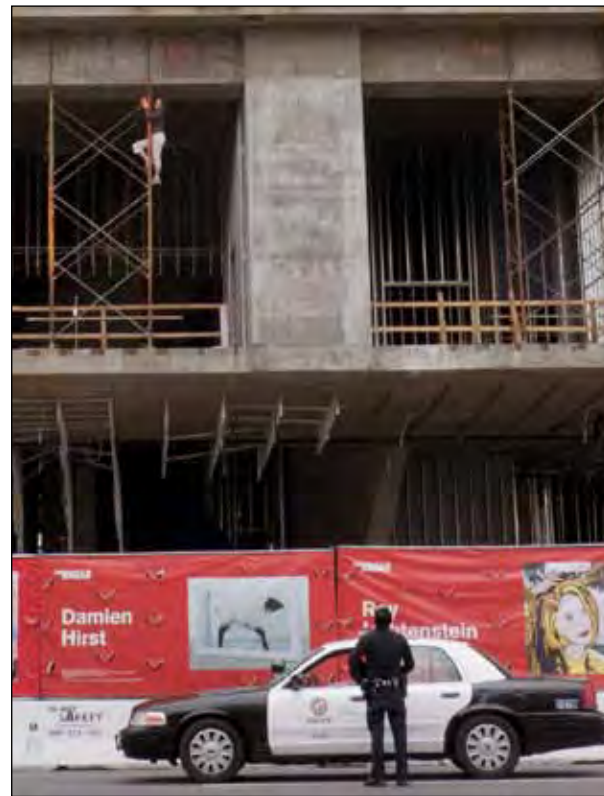
Untitled (Street Performances) Broad Museum Construction Site, Los Angeles February 10th, 2013 Mason Line; Photo: Sandra de la Loza
